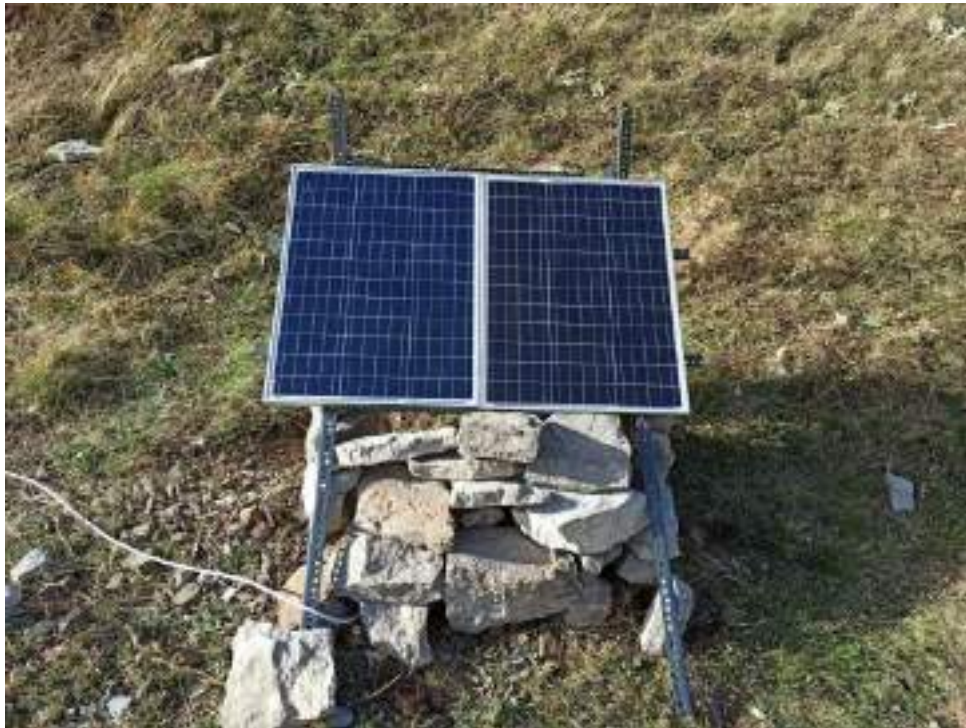
Figure 18. Solar Panel for power sourcing the device.
